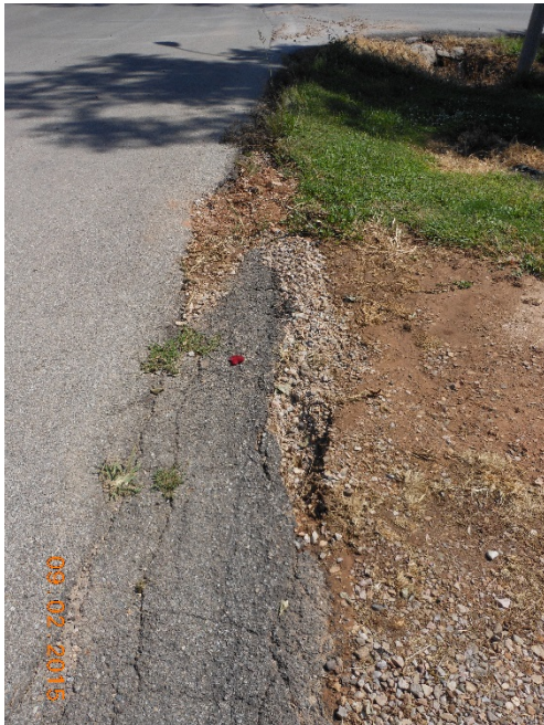
Photo 3. Edge Erosion at Filled Ditch
