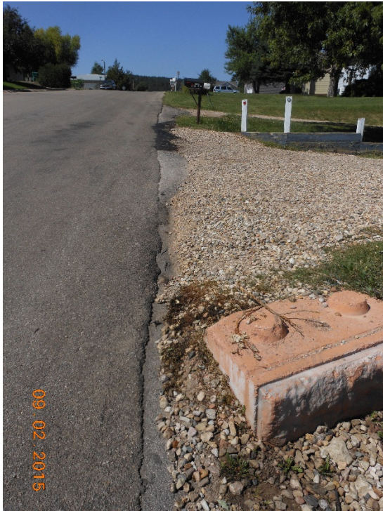
Photo 5. Edge Rut Erosion Due to Landscape Feature
