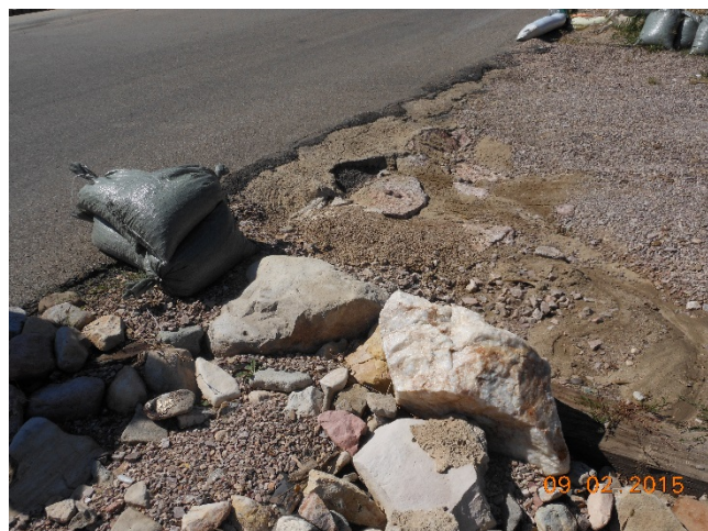
Photo 4. Sandbagged Drainage Erosion at Driveway Caused by Diverted Flow
