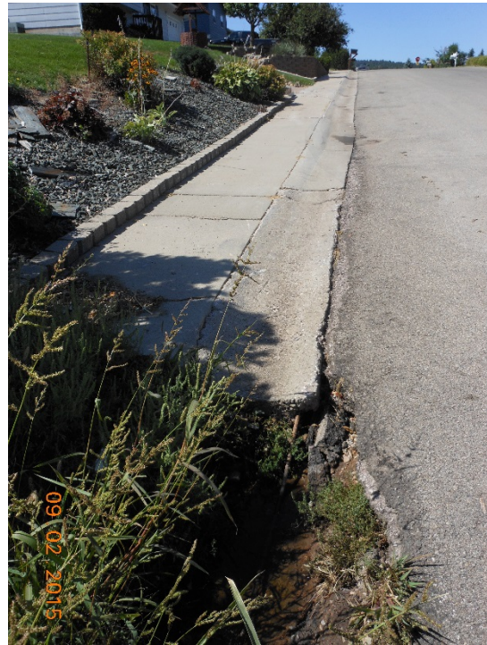
Photo 6. Erosion at End of Gutter Pan
