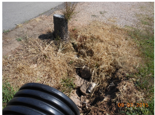
Photo 8. Erosion at 24" Pipe Discharge
