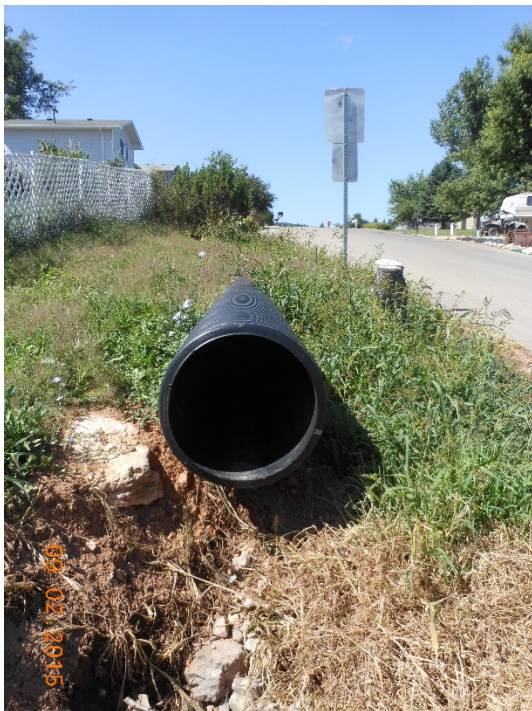
Photo 7. 24" Elevated Discharge Pipe
