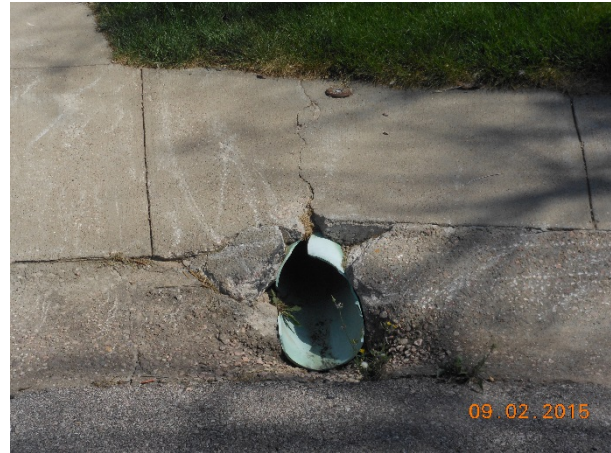
Photo 10. 10 " Diameter Storm Inlet on Maple Drive
